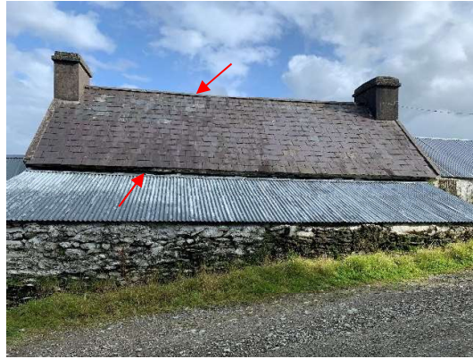
2. Rear view of dwelling indicating potential access points in raised ridge tiles and soffit
