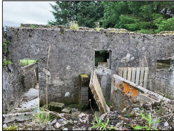
Plate 3-1: Example of derelict buildings present at Inchamore
